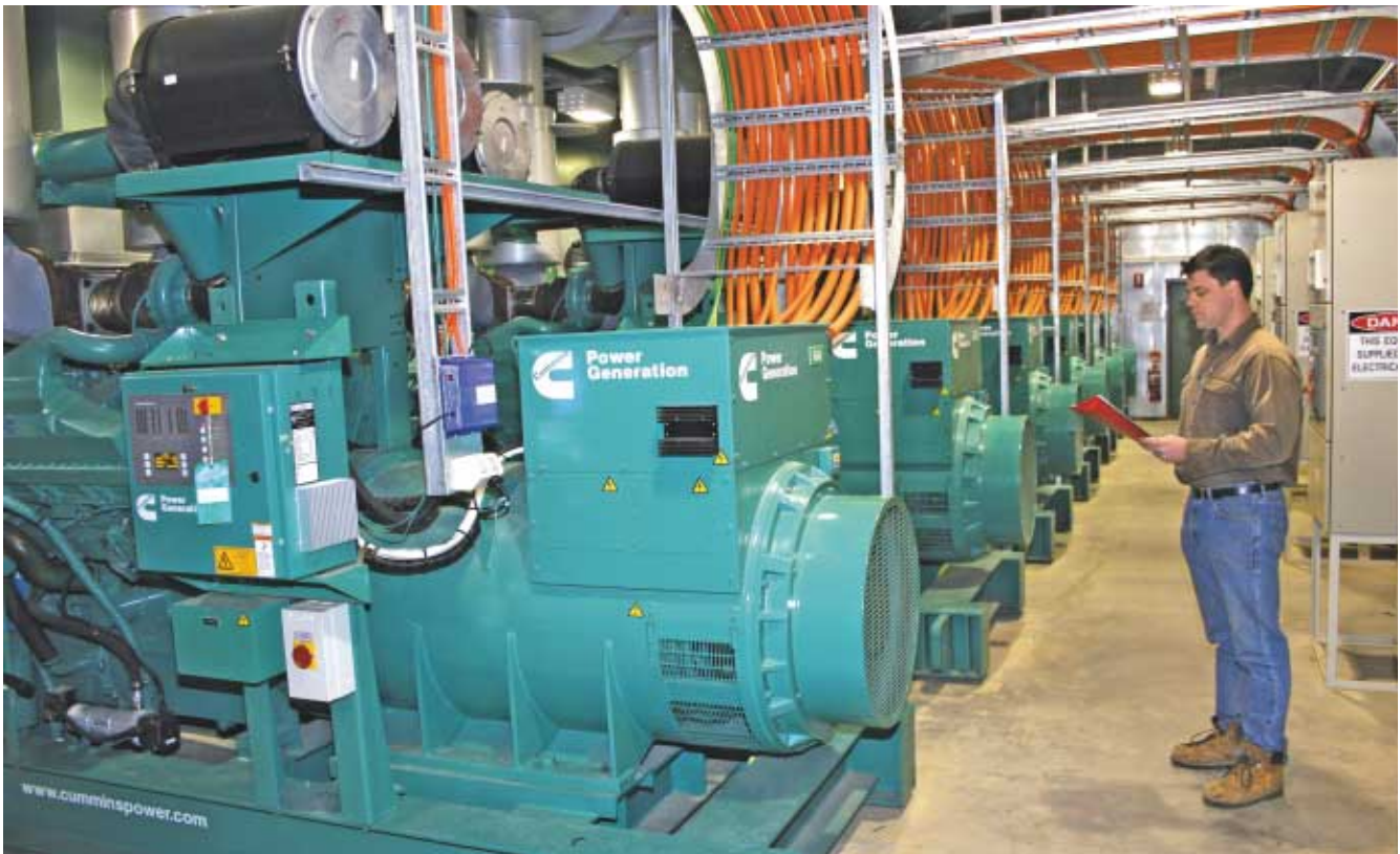
Inside one of the three buildings that houses the diesel generator sets
